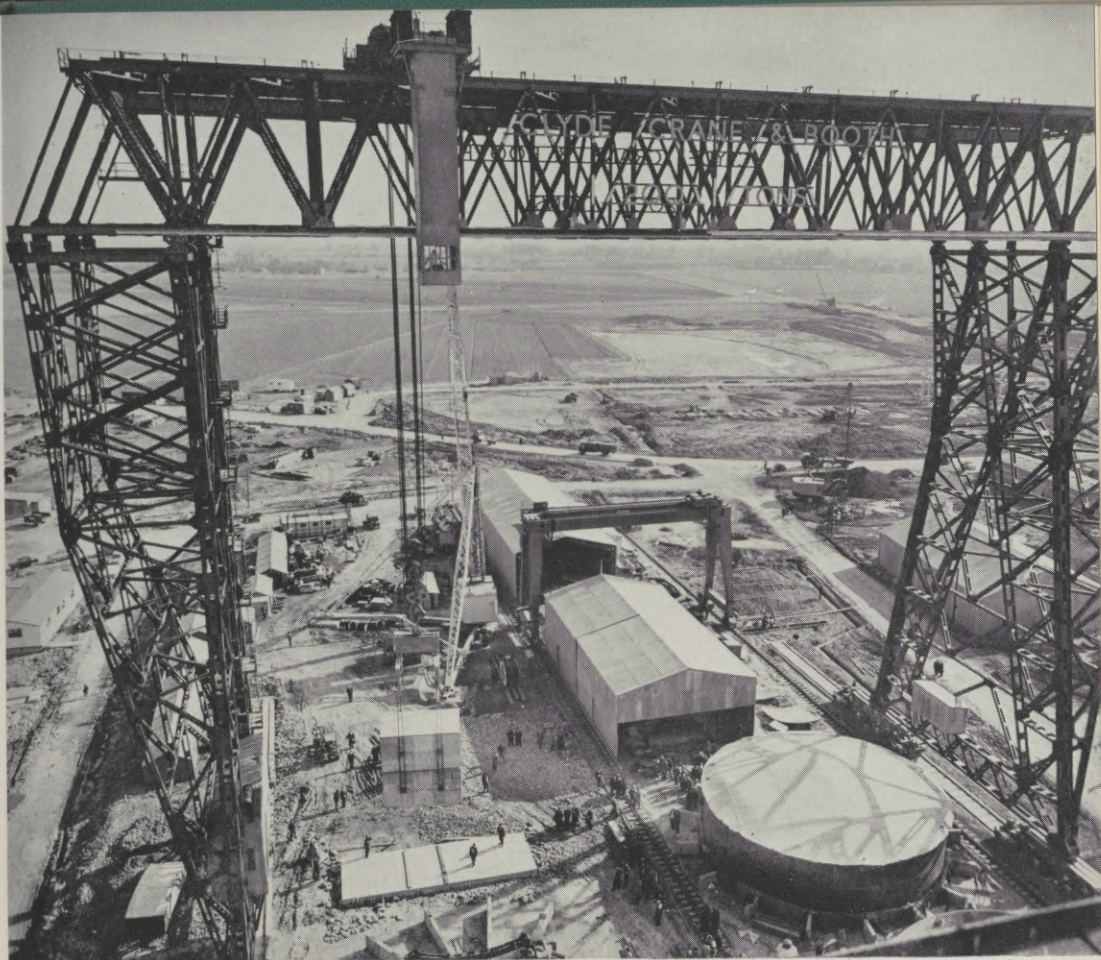
Goliath giant crane, capable of lifting 200 tons, being used to build Bradwell nuclear power station.
