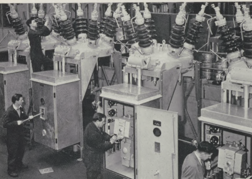
Outdoor oil circuit-breakers being checked at the English Electric Company works at Stafford before shipment to Los Angeles.
