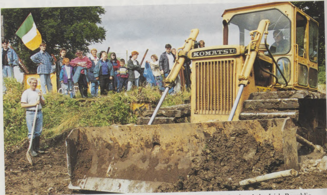
A bulldozer clears a path through a barrier on the border of Northern Ireland and the Irish Republic, reopening a crossborder road closed for the last 25 years for security reasons.
